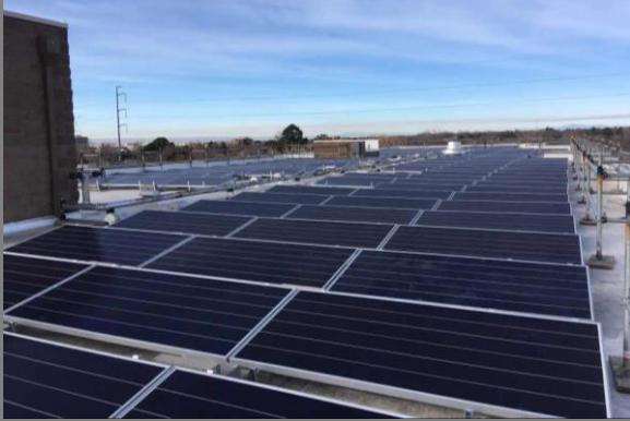
Albuquerque Housing Authority Rooftop Solar
