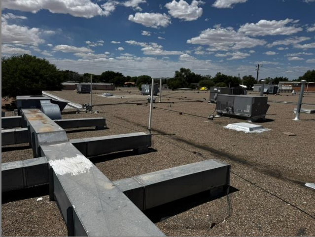
Aging HVAC Infrastructure
