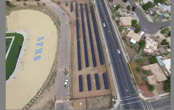
Santa Fe High School 1MW Solar array
